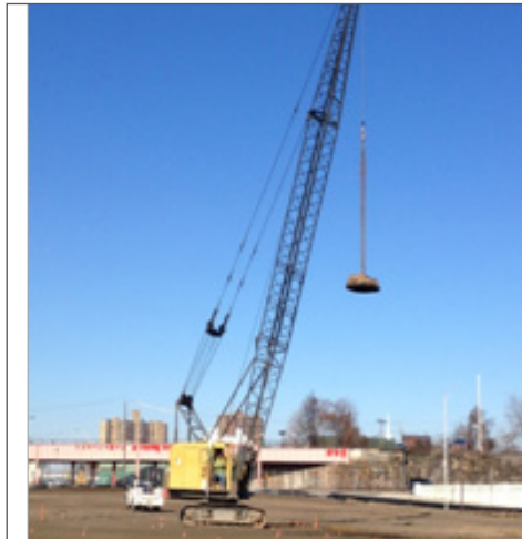
Soil improvement using DDC (DDC crane dropping weight and DDC weight generated craters).
